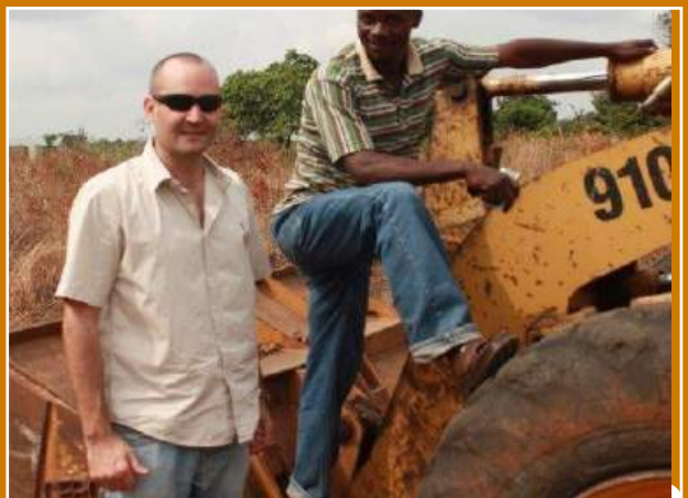
Dirk Kotze (T4D) on site where groundworks are being done for the erection of a new learning facility in Tanzania
